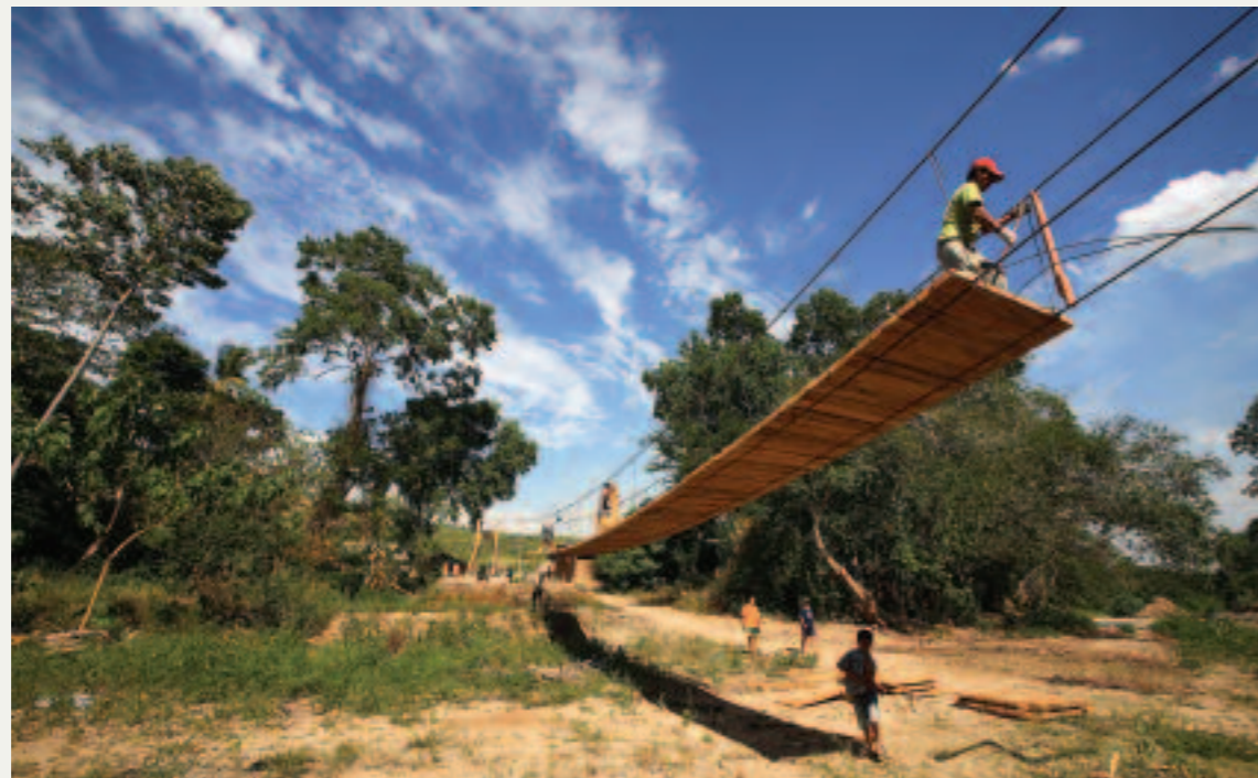
Above: Construction of the wooden footbridge deck. Below right: The bridge towers being erected
